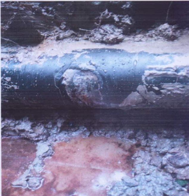
Fig C: The Leak Point after excavation
